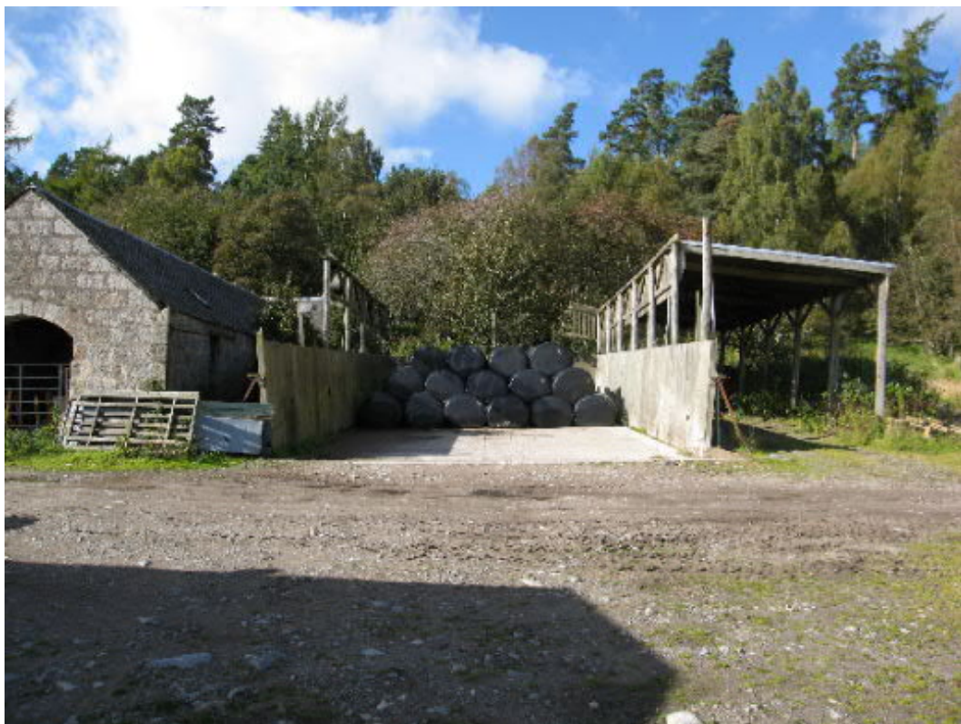
Brownfield site from East. Central roof structure missing due to storm damage
